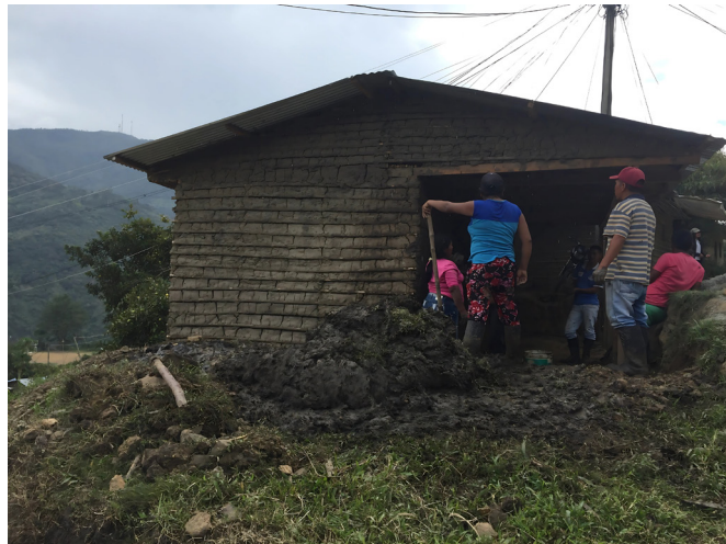
Construction of a traditional dwelling in the Indigenous Resguardo of Toribío, Cauca. © Julián Ruiz, 2016. Personal archive.
